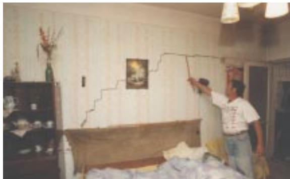
Checking the damage caused by the River Tisza flood in 2000
